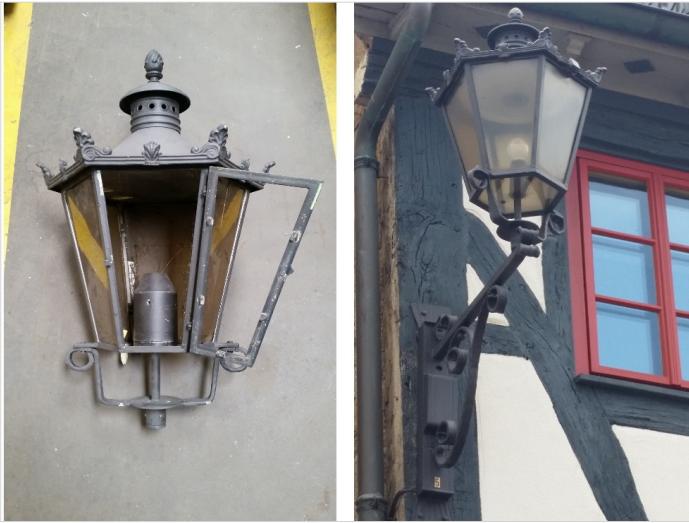
Before the retrofit: Desolate condition of the existing luminaire body
